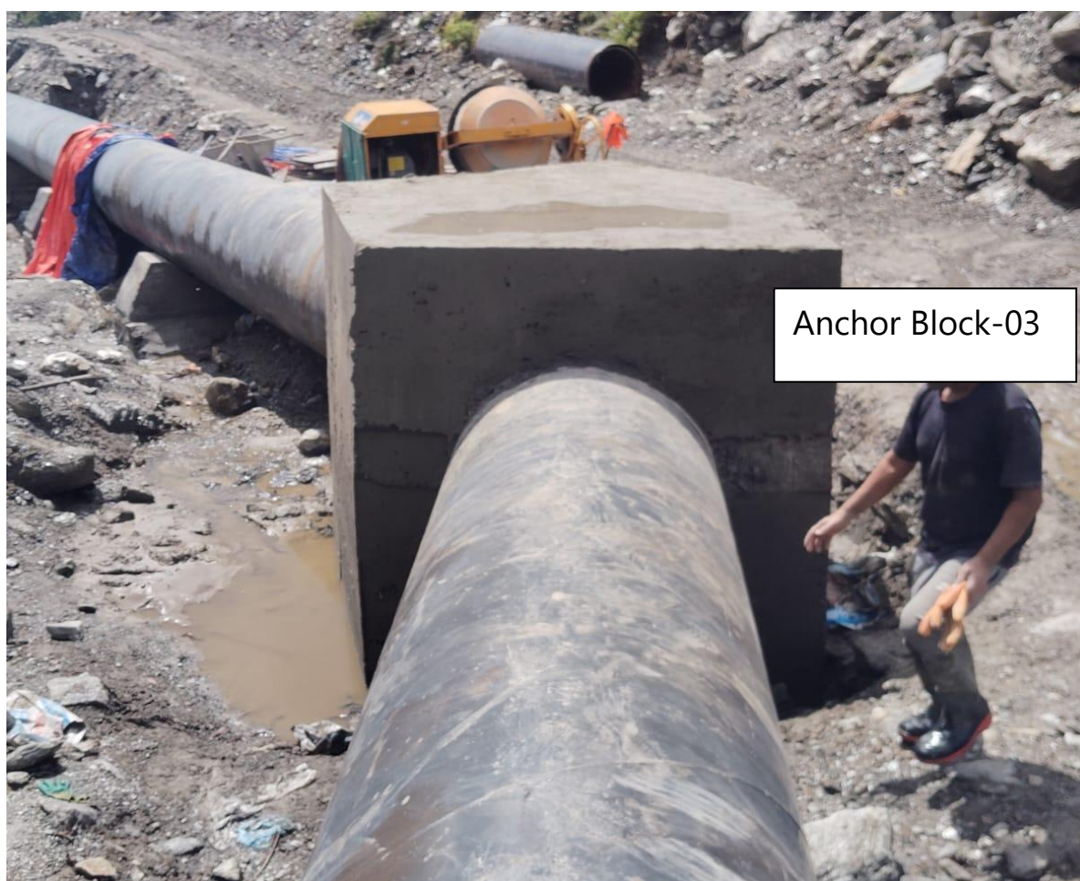
Figure 6: Headrace pipe Anchor blocks.
