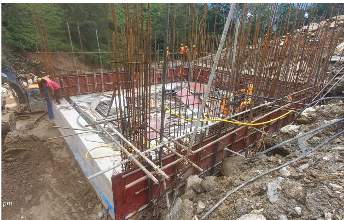
Figure 10: Powerhouse machine hall bay-02
